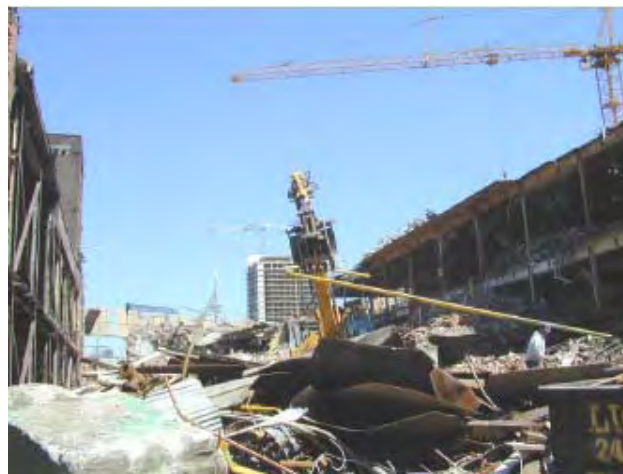
The Irwin Toy warehouse is being remade into a place to “live, work and play.” Looking west through the partly demolished building.
